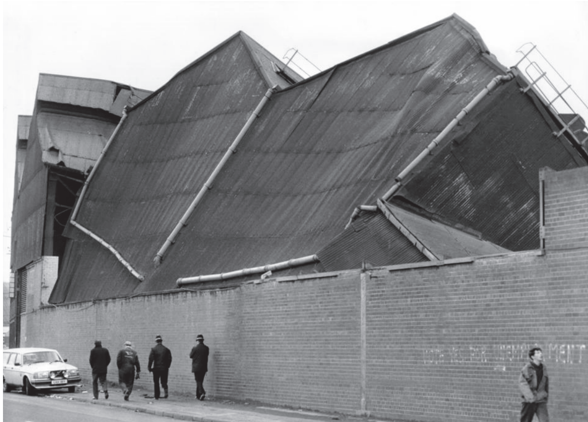
Figure 15 Gale damage Savile Street East 26 th February 1990 (courtesy Sheffield Newspapers)
