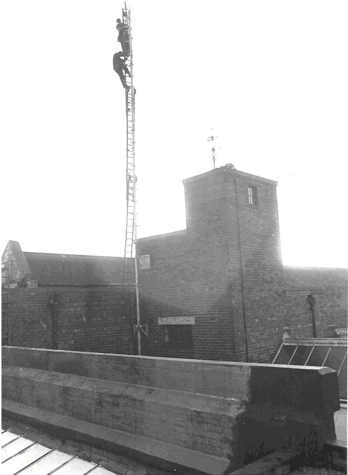
Figure 28 Dismantling of the Dines anemograph mast in January 1980 by Harrisons steplejacks to make way for the Munro electrical anemograph mast (© Museums Sheffield)
